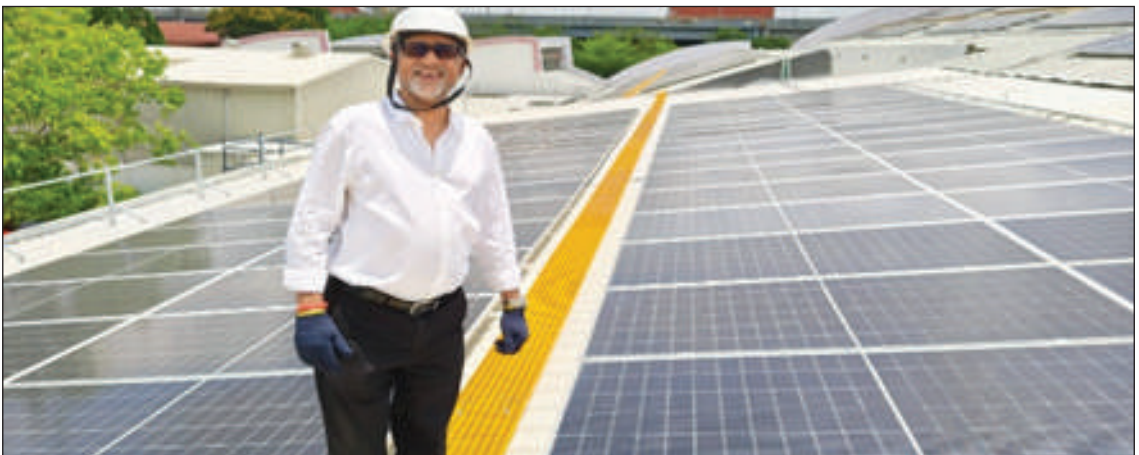
205 kW Solar Power Panel Installed at the factory
