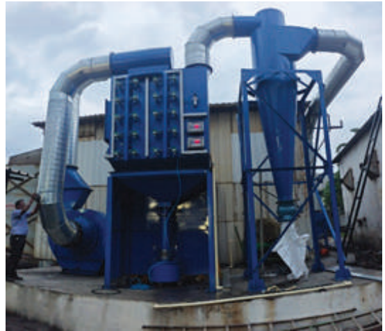
Addition of New Dust Extraction Unit
